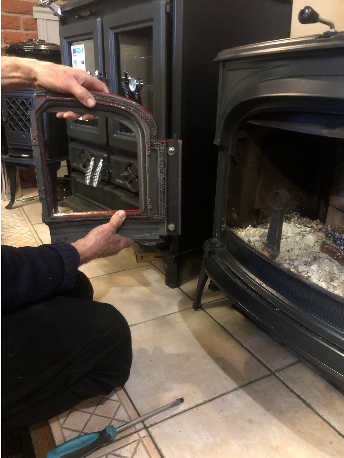
Figure 3 Door is free from stove with clamp and fasteners clear to see.
