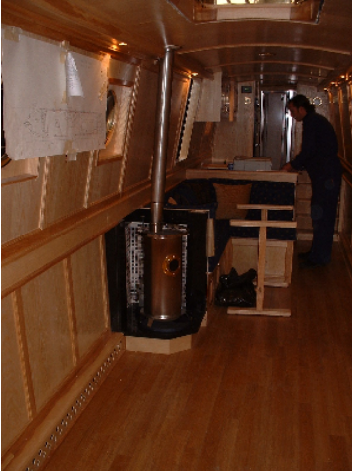
SHED STOVE ON GRANITE AND TILE FIREPLACE (INCORRECT FITTING)
